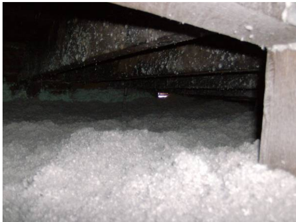
Blown Cellulose in Attic
