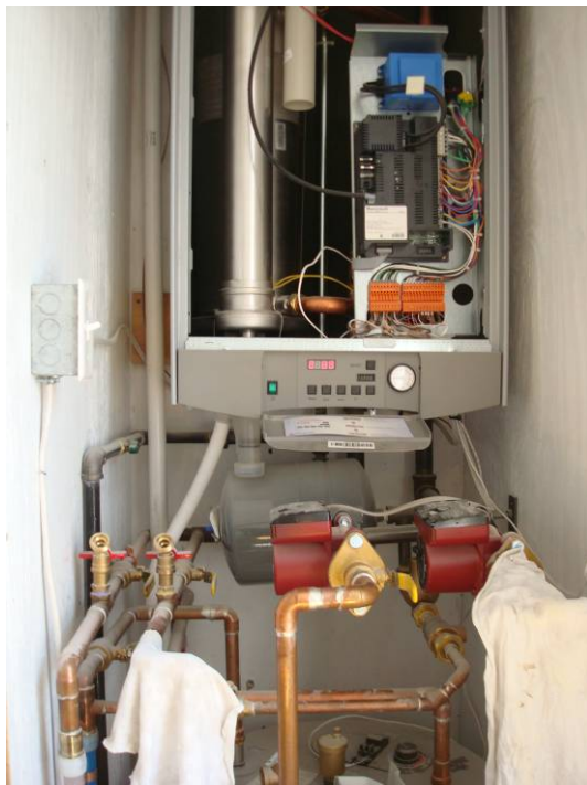
Wall Hung Boiler located in the Bathroom of each Apartment
