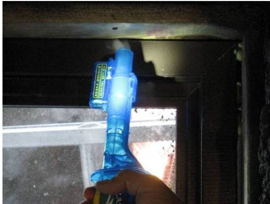
Air leak at top of window
