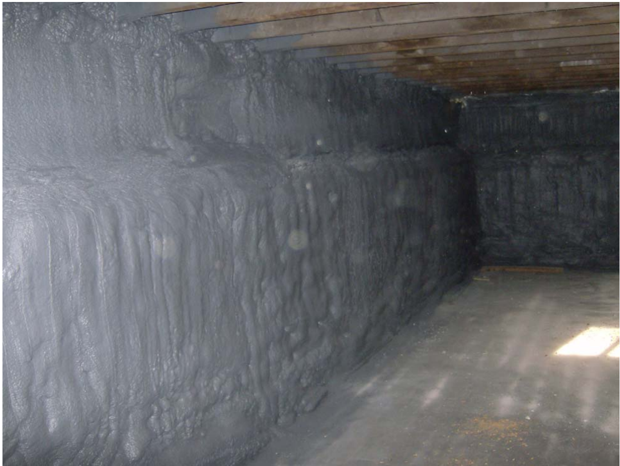
Figure 4. Closed Cell Insulation on Basement wall with EPDM Membrane on Basement Floor
