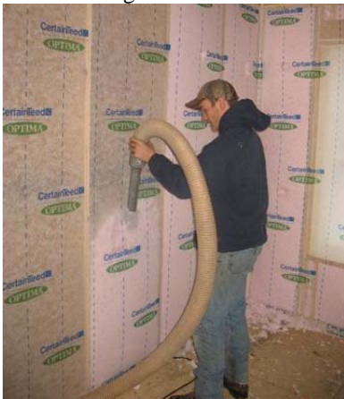
BIBS System in Exterior Wall
