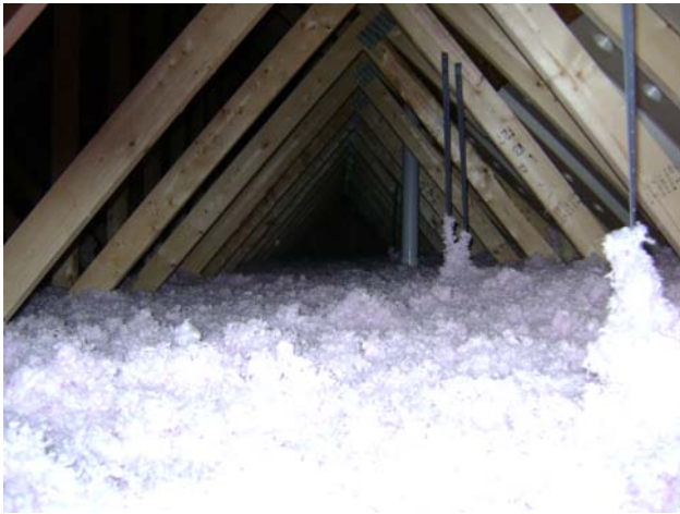
Blown Fiberglass in Attic
