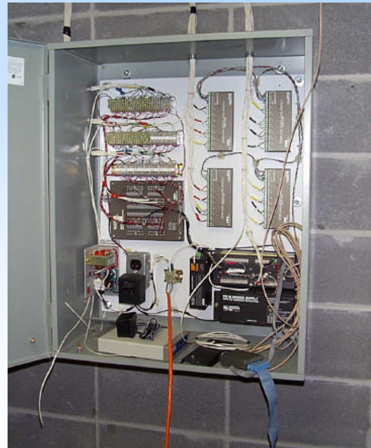
Data Logger B - Pod Areas
