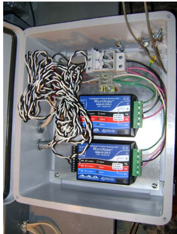
Power Transducers installed near electric panel
